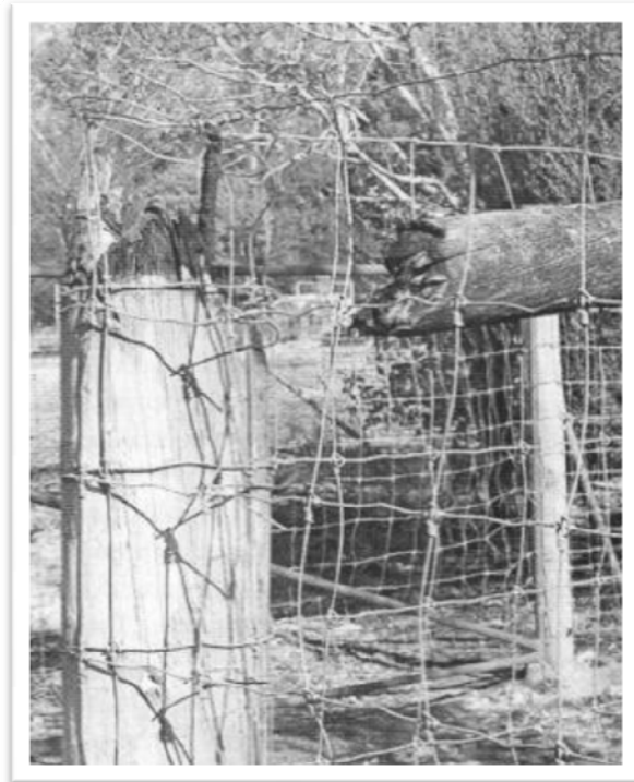
Partially burnt strainer assembly
